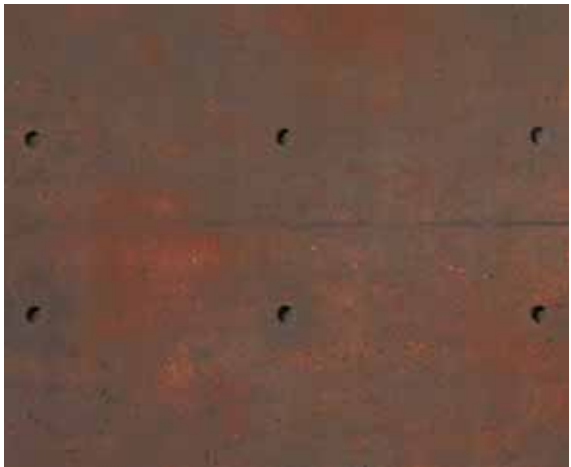
M-172 Rusty Concrete Wall Panel
